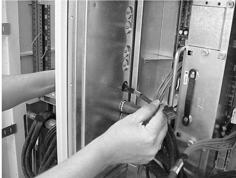
Figure 3-41 Passing the GSP Bus Cable Through the Cable Exit Panel
