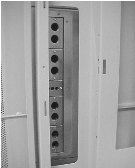
Figure 3-20 IOX Cabinet Alignment (Rear)
