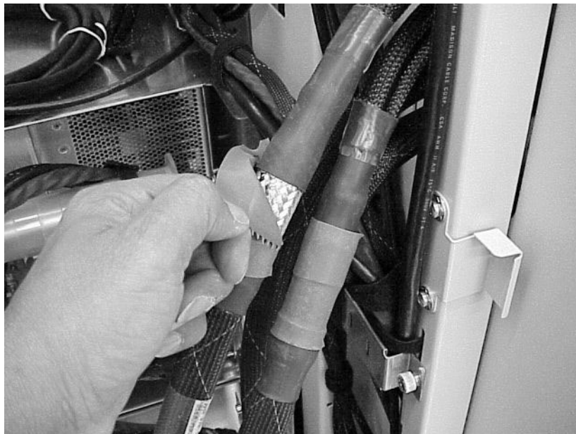
Figure 3-34 REO Shield Exposed
