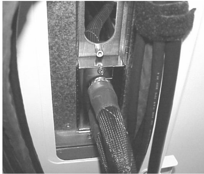
Figure 3-37 REO Cable Pair Mounted in R-PEC and Installed in Cable Exit Panel
