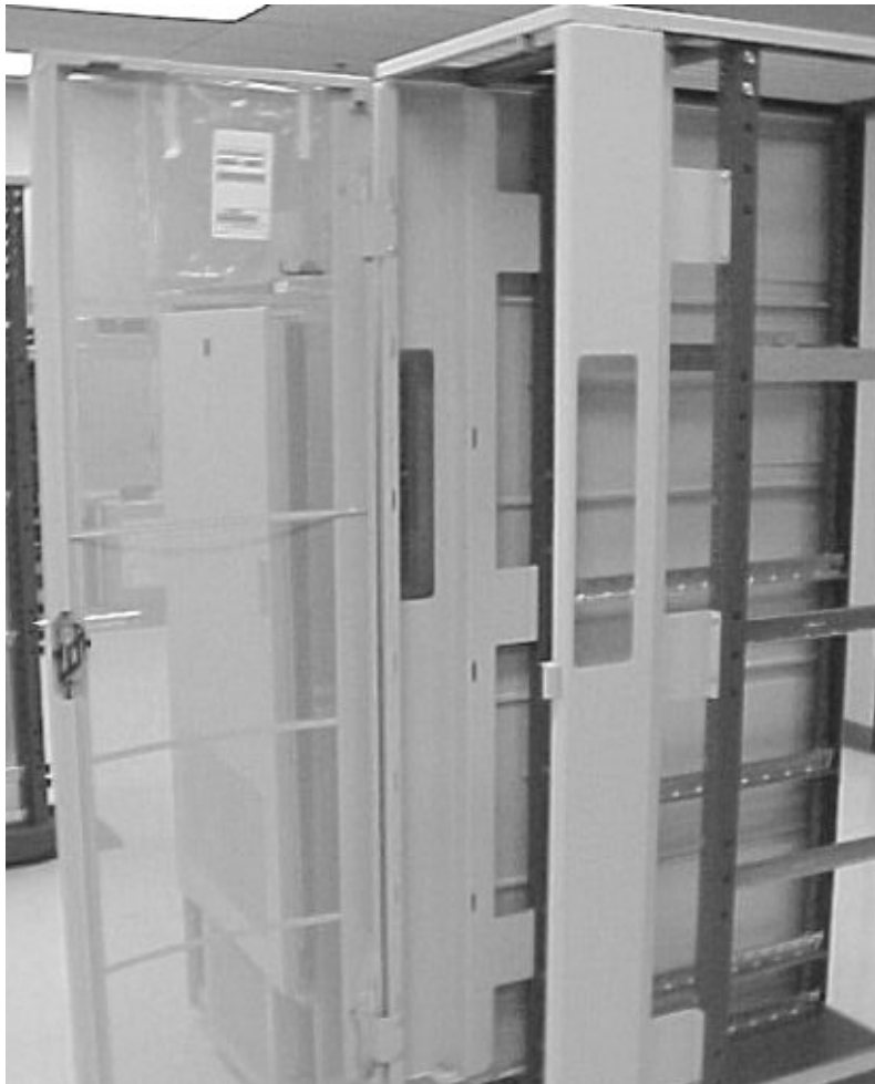
Figure 1-17 IOX Cabinet (Rear View)
