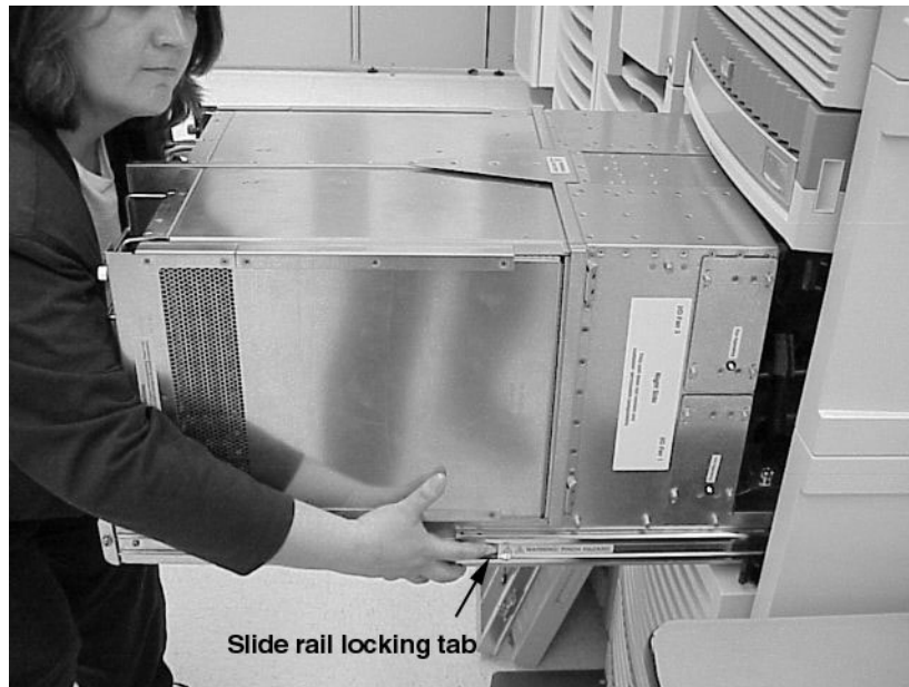
Figure 6-11 Pushing the ICE into the Cabinet
