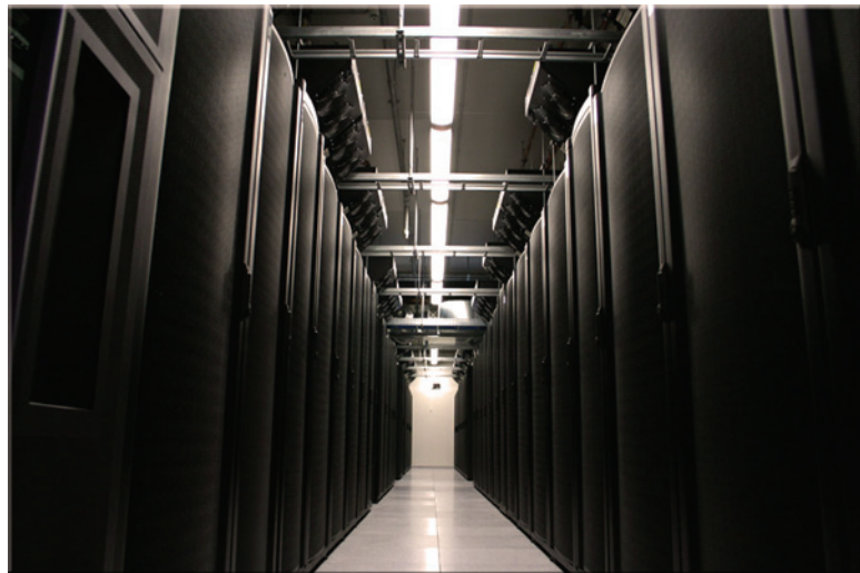
Figure 29. Our Prague datacenter was built to operate within the constraints of the building. It achieves the highest square footage density of all of our datacenters, with an average of only 26 ft 2 per rack.
