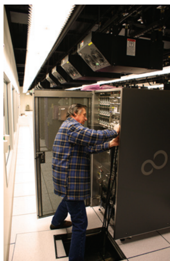
Figure 24. The Sun Solution Center in Menlo Park, California is designed to have a neat and clean appearance using the same modular design combined with a raised floor for power and connectivity access.
