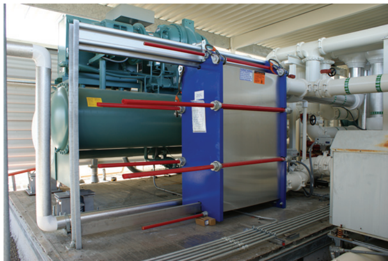
Figure 27. A water-side economizer uses outside air to directly chill the cooling system's water when outside air temperatures are sufficiently low.
