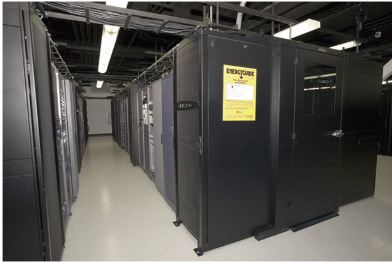
Figure 17. Pods cooled with hot-aisle containment and in-row cooling have an unmistakable appearance.
