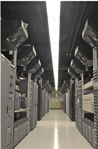
Figure 20. Overhead Liebert XDV top-cooling modules can be used in open environments.
