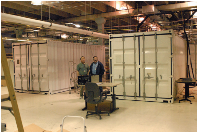
Figure 31. Two Sun Modular Datacenter S20 containers used for testing at our Louisville, Colorado facility were installed in three weeks.
