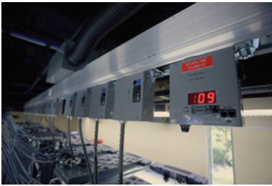
Figure 13. Modular busways provide flexible, adaptable power distribution that is monitored and can be changed rapidly.
