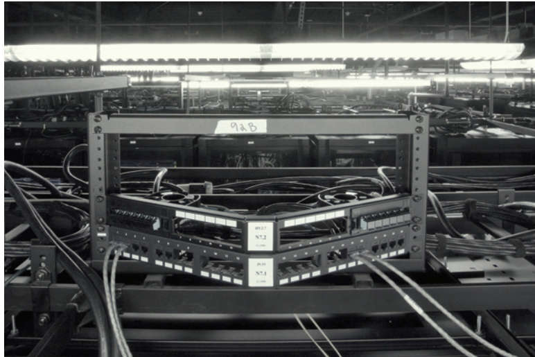
Figure 21. Patch panels above each rack position support a wide range of connectivity requirement while providing room for future expansion.
