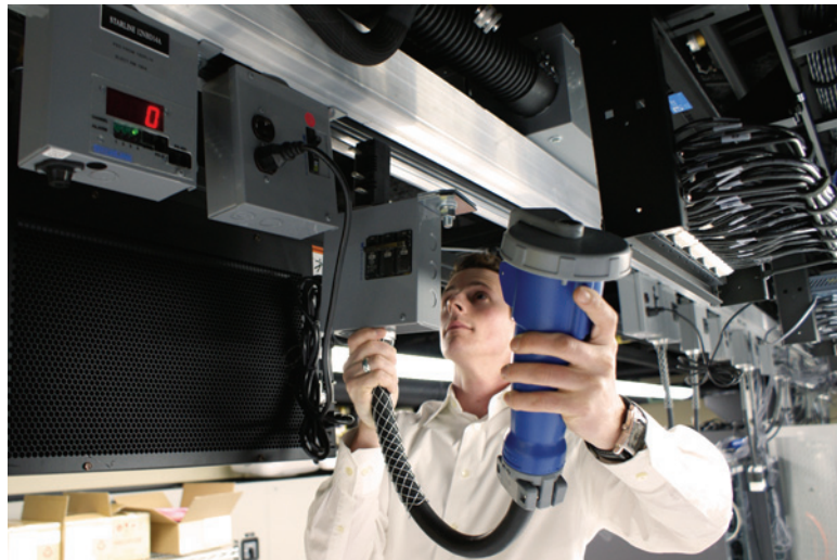
Figure 14. The Starline busway supports an intermixing of 120V, single-phase up to 208V, 100A, three-phase power feeds. In this example, a 60A three-phase can is being plugged in beside a 120V can.
