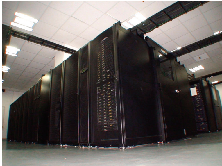
Figure 30. Our Bangalore datacenter was built to operate within the constraints of leased office building space. It uses hot-aisle containment, and fits within the office building's standard ceiling height.
