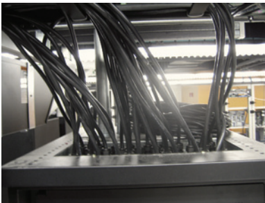
Figure 12. Using PDUs can result in an unmanageable snarl of cables. Pictured are whips running from a PDU to an overhead cable tray.
