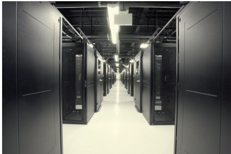
Figure 22. The Santa Clara Software datacenter has 18 pods based on in-row cooling and hot-aisle containment.
