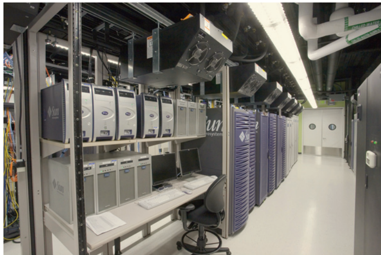
Figure 23. The Services organization datacenter required a high degree of flexibility, with lab benches and racks. This was an ideal application of the Liebert XDV cooling modules.
