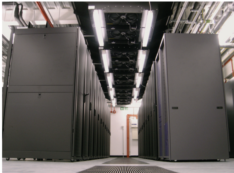
Figure 28. A customer-facing datacenter at our Guillemont Park campus in Blackwater, U.K. uses a combination of ambient cooling using a raised floor and Liebert XDO cooling modules that are positioned over the cold aisle.
